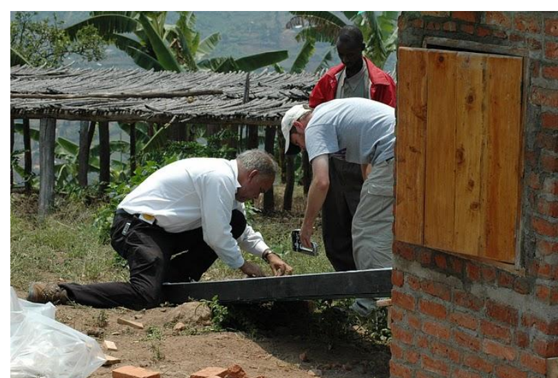
Jack and Chris working on the solar collector for the prototype fruit dryer
